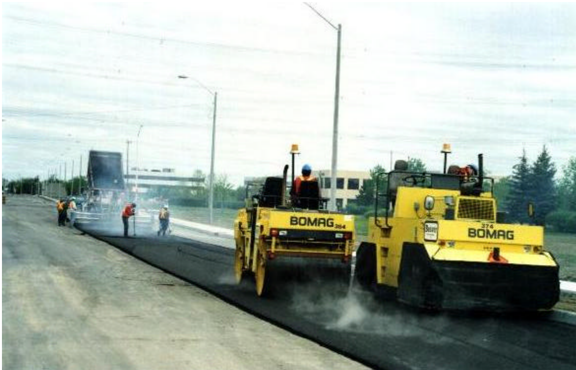
PHOTOGRAPH 4: Compaction Equipment Rolling Hot Mat. Note Heating Vent and Skirts on Rubber Tired Roller to Aid in Preventing Pick-up.
